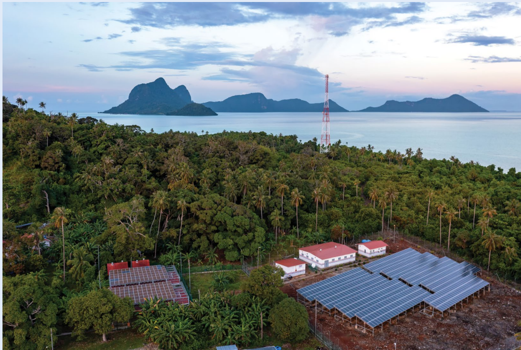
Figure 4.7: Several buildings are using this micro-solar grid on Selakan Island in Malaysia.
